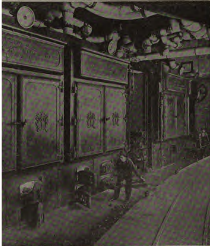
D—FURNACE ROOM OF THE CHICAGO PUBLIC LIBRARY.
